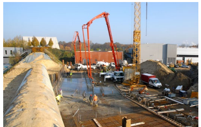
FLASH 2 construction in November 2011. Meanwhile this part is completed, the old tunnel (on the left, with the experimental hall in the back) covered again with sand and the FLASH 1 FEL is back in operation. http://flash2.desy.de
