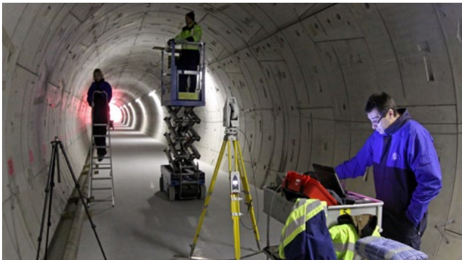
Survey works in February 2012 in one of the future undulator tunnels of the European XFEL after completion of civil construction.
